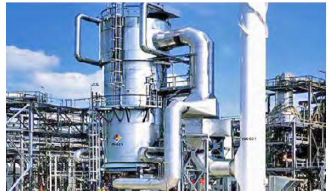
| A bottom-fired heater 32 MW for Petro in DE
